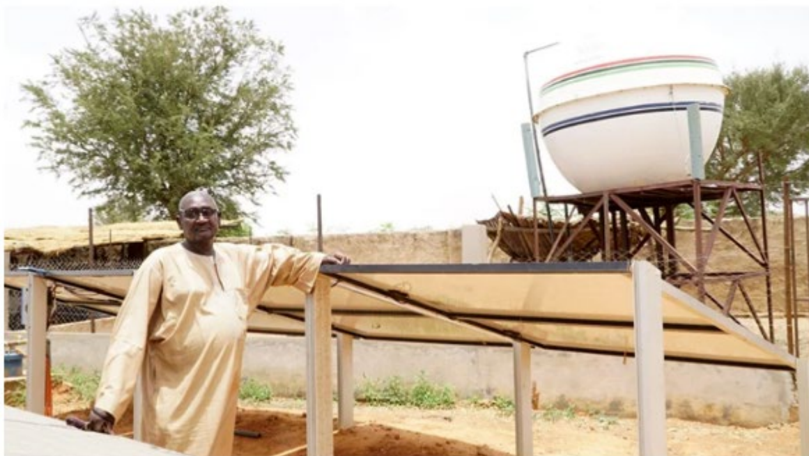
Boubacar Issoufou Alzouma stands beside solar panels. The solar-powered water pumping system enables Alzouma to rotate crops on his farm in Finaré, Niger.
